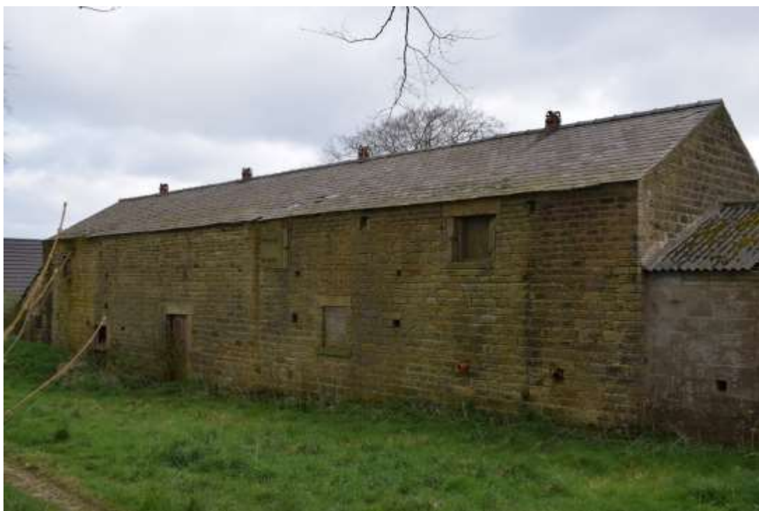
Fig 24. The rear (western) roof pitch showing the strap repairs and the lichen bloom
