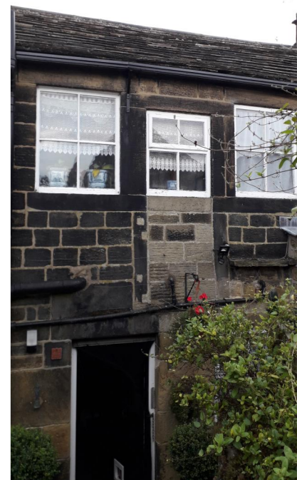
Existing external door to be covered up due to extension but left in place to aid as draft lobby when extension is in place
