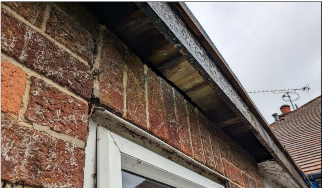
Plate 9. Missing soffit panel on garage
