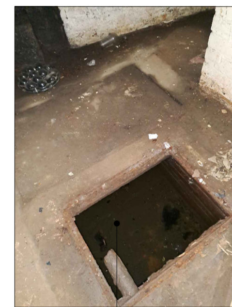
Assumed sump inspection chamber in basement of No.303 - Requires investigation - Refer to Photos 30 to 32 for further details
