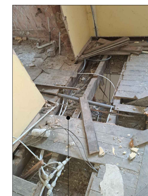
Indication of suspended first construction in disrepair above ground floor accommodation (certain areas)
