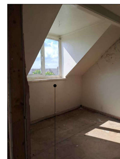
Indication of typical second floor dormer attic flat window facing Barnsley Road
