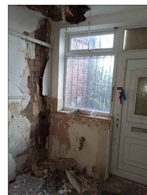
Indication of existing construction in disrepair to ground floor flat accommodation to rear of building (straddles No.305 & No.307)
