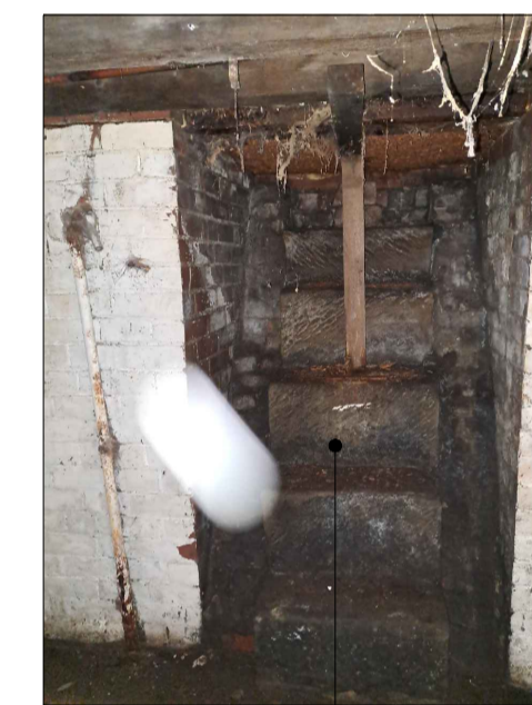
Stone steps forming staircase - assumed to be from basement to covered access (blocked up)
