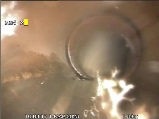
Photo: 42_4a, 00:00:00 1.9m, Joint displaced. Medium
