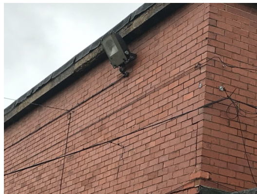
Image 6: Lifted felt on western side of Building 1
