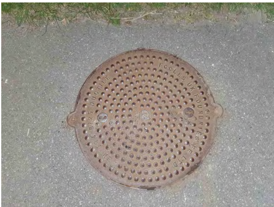
SW2 UTR Bolted Cover Seized
