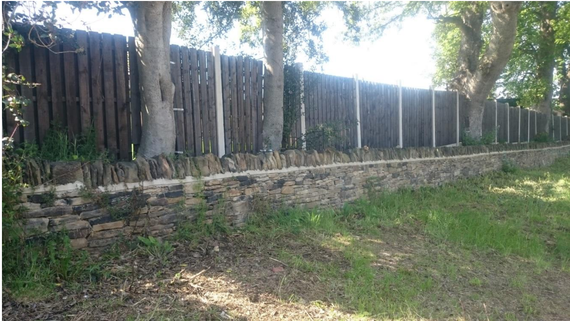
Photo 3. Showing the retaining wall on east side of the stems of trees 023 (left), 024, and 022 (right). The land behind this wall, on which the trees are growing, is raised by 500 to 600 mm.
