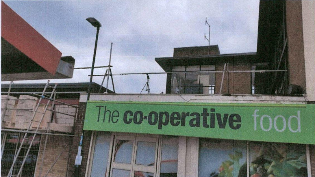
Picture 3: Measurements to the side of Hoyland Town Hall facing Hoyland Market and above the Co-operative food store. This measurement location is labelled ML3.
